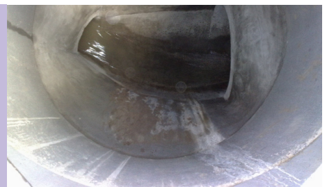
Upgraded inlet pipe
