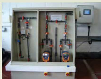
Castlemartin chlorine dosing
